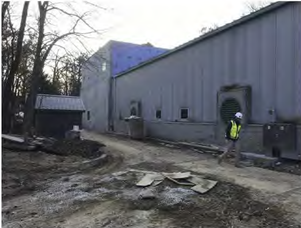
Photo #11. Service road running on the east side of the Elephant Barn. New 50 foot addition is at the southern end of the barn.
