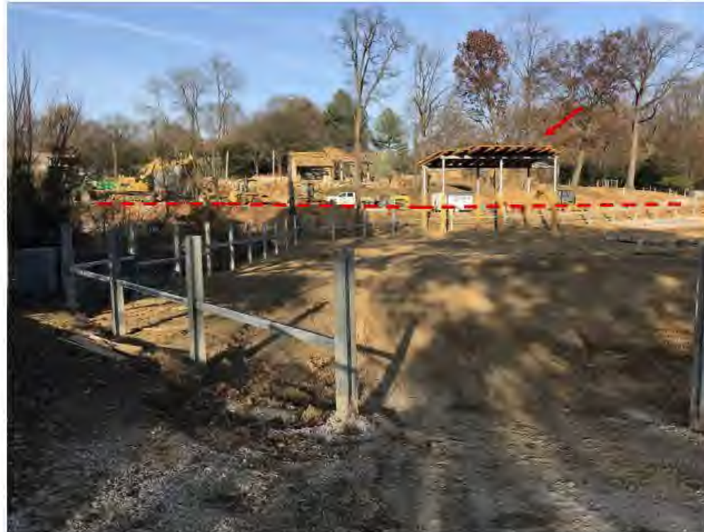
Photo #1. View of Savanna flex exhibit-giraffe and elephant will be able to share this exhibit. Red arrow indicates location of elephant shade structure. Red dotted line indicates location of guest viewing. Landscaping will be added around the exhibit in the Winter of 2018 and Spring of 2019.
