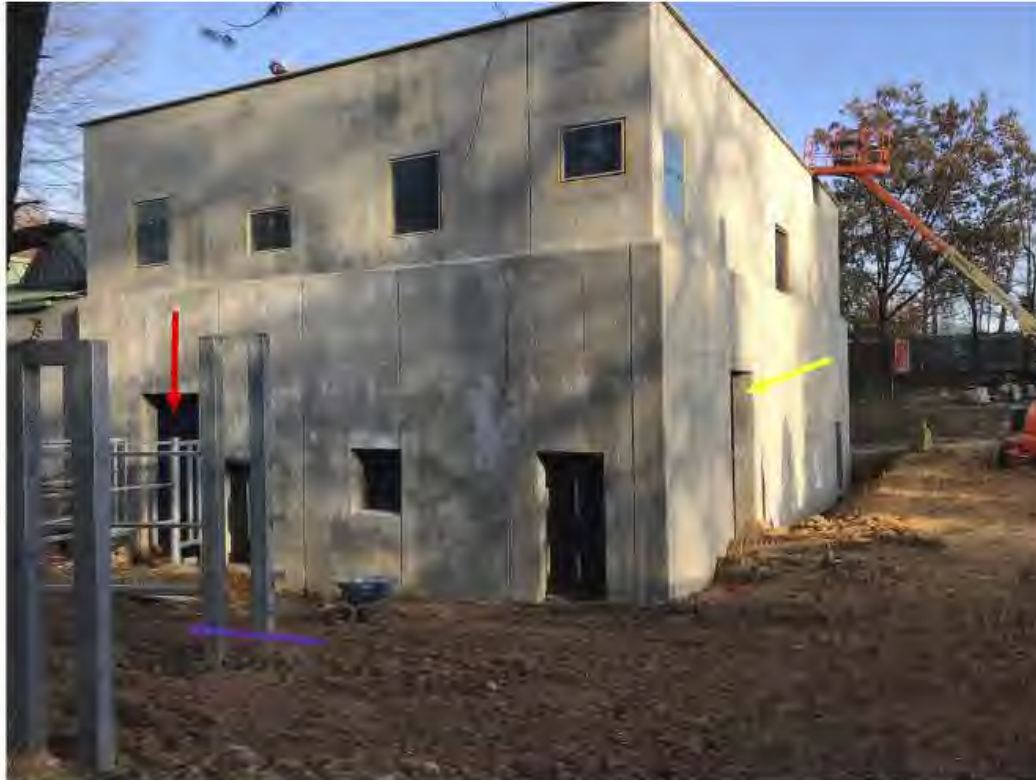
Photo #10. Western and southern faces of the new 50 foot addition to the elephant barn (currently under construction). Red arrow indicates location of chute into the addition from the Valley Habitat. Area to the right of the building is the boma yard, an off exhibit holding area. Purple arrow indicates chute from the Valley Habitat into the boma yard. Yellow arrow indicates doorway into the addition from the boma yard.
