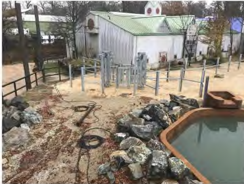
Photo #8 View from guest viewing deck of transfer chute between Forest Yard (on the left) and Valley Habitat (on the right).
