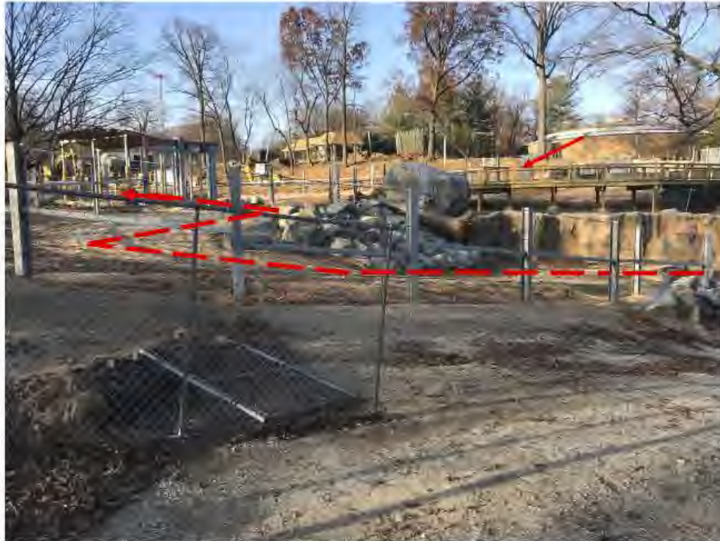
Photo #3. View of Savanna passage exhibit. The function of this exhibit is to give the elephants a means of moving from the exhibits by the elephant barn to the new Savanna flex exhibit. The elevation of the Savanna flex exhibit is roughly 14 feet higher than the other elephant exhibits. Savanna passage is a switchback (222 feet long) that allows the elephants a means to safely walk up to the new elevation. Red arrow indicates location of guest viewing deck that overlooks the Savanna flex exhibit. Red dotted line roughly indicates how the elephants will move through the exhibit.
